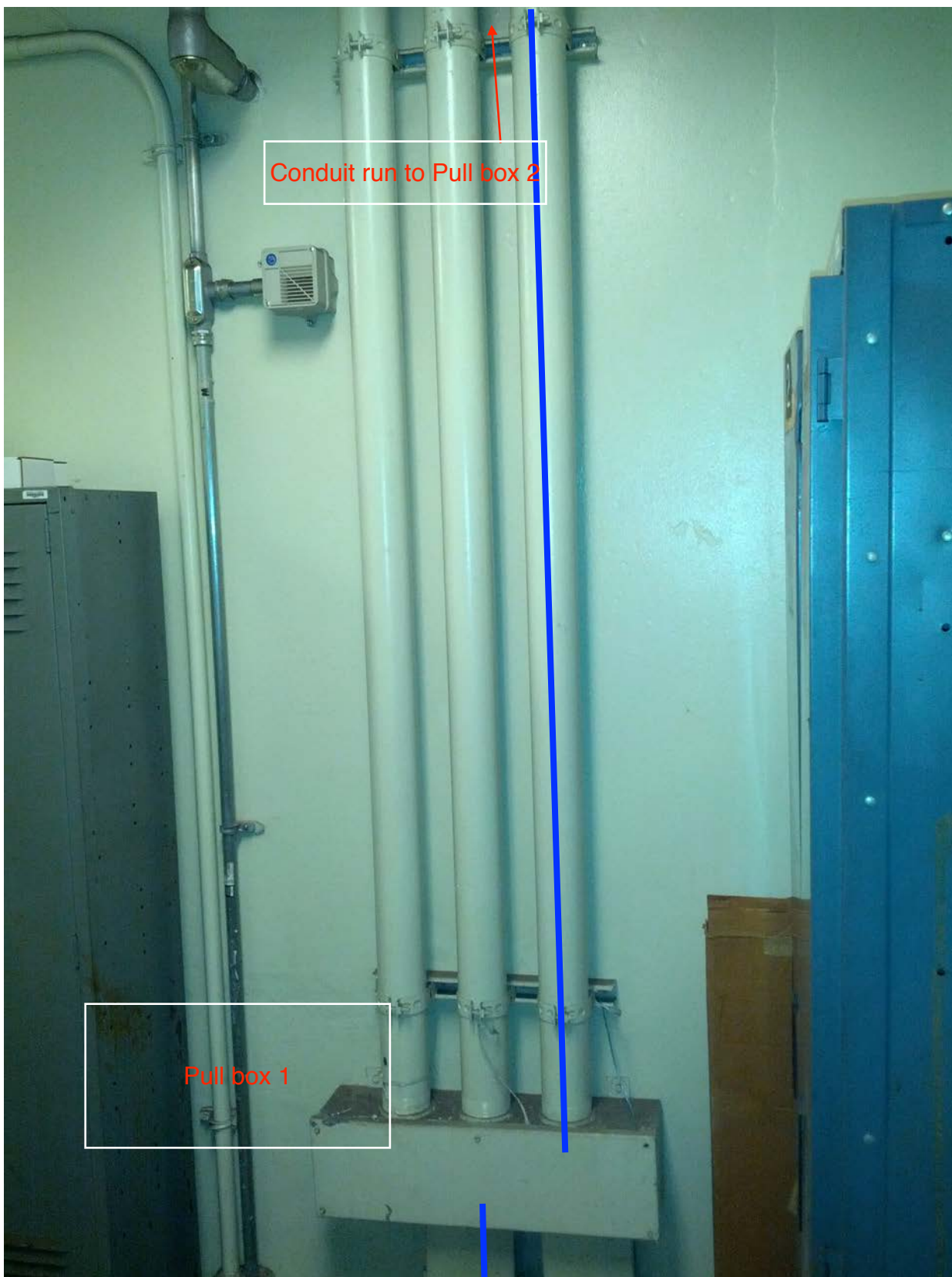
Photo #5 – E02 Shaw-Howard U South: Pull box 1 to Pull box 2
