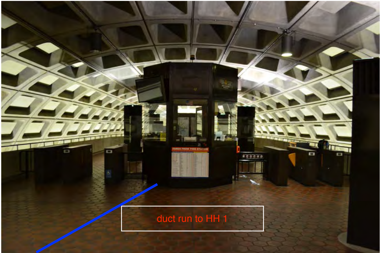
Photo #1 – E02 Shaw-Howard U South: Kiosk to Handhole 1
